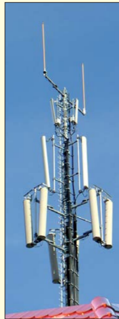
Cell Phone Antennas on Rooftop of House
